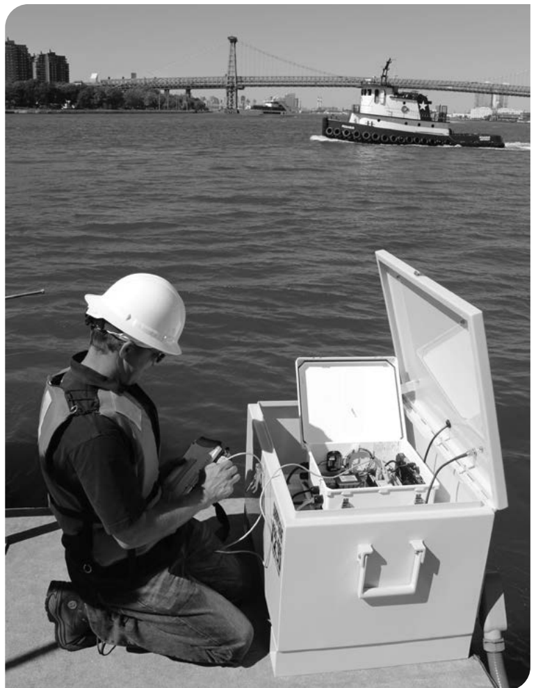
An example of a NEMA enclosure where the DCP Signal Output Adapter is wired.
